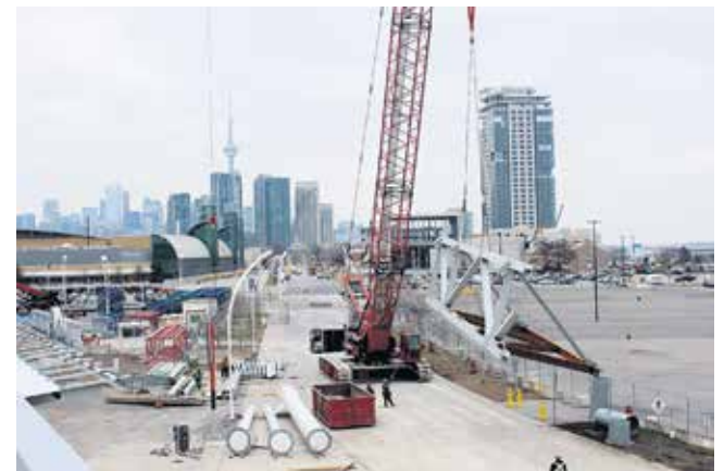
Crawler works on BMO Field renovation with Toronto city skyline as a backdrop. Photo courtesy of PCL Constructors Canada Inc.
