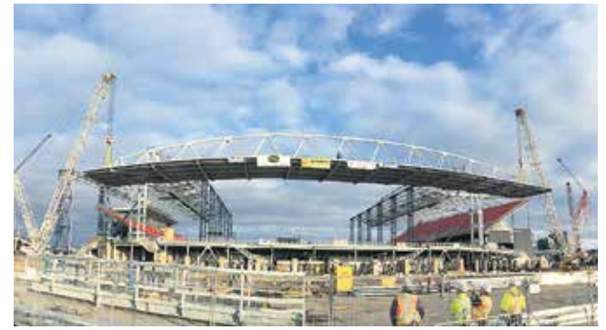
Camera captures wide-angle view of tandem lift of roof canopy during renovation to Toronto's BMO Field. Photo courtesy of PCL Constructors Canada Inc.
