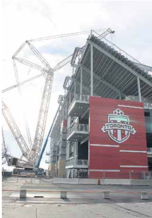
Stadium is the home pitch of Toronto’s North American Soccer League club. Photo courtesy of PCL Constructors Canada Inc.
