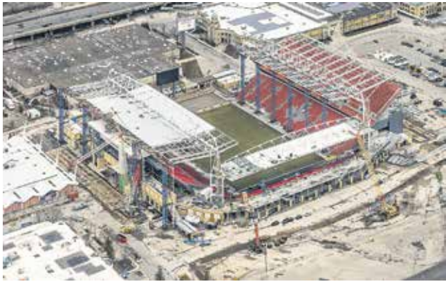
Aerial view shows progress on crane work during renovation of BMO Field. Photo courtesy of PCL Constructors Canada Inc.
