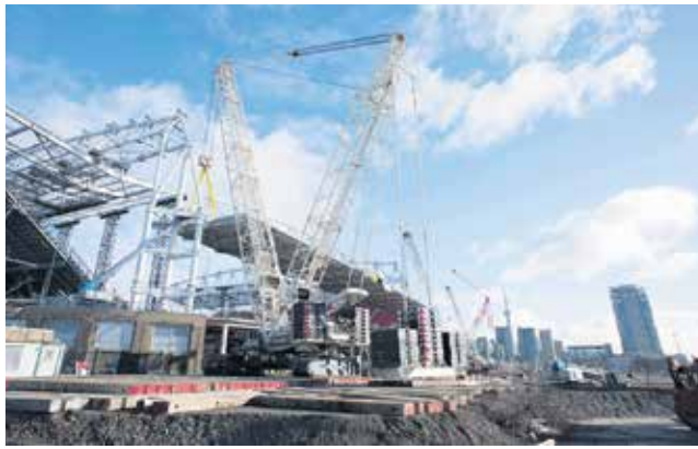
Mammoet Canada Eastern uses two Demag crawlers to install a canopy at Toronto's BMO Field. Photo courtesy of Canam-Heavy
